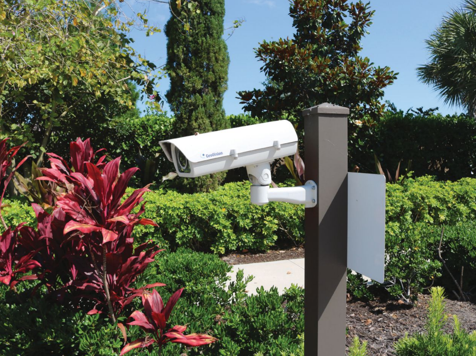
Photos courtesy of Envera Systems
